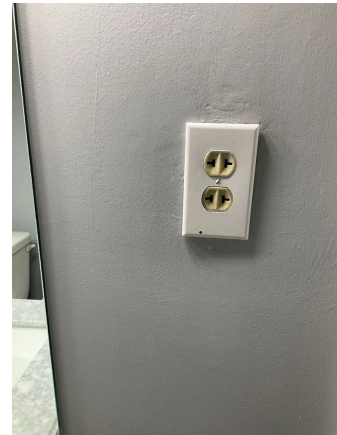
Two prong outlet noted
