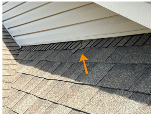
Minor loose trim shingle noted over carport
