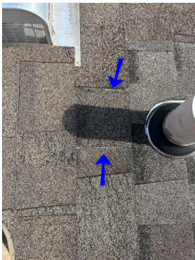
Sealant noted that vent boot penetration area
