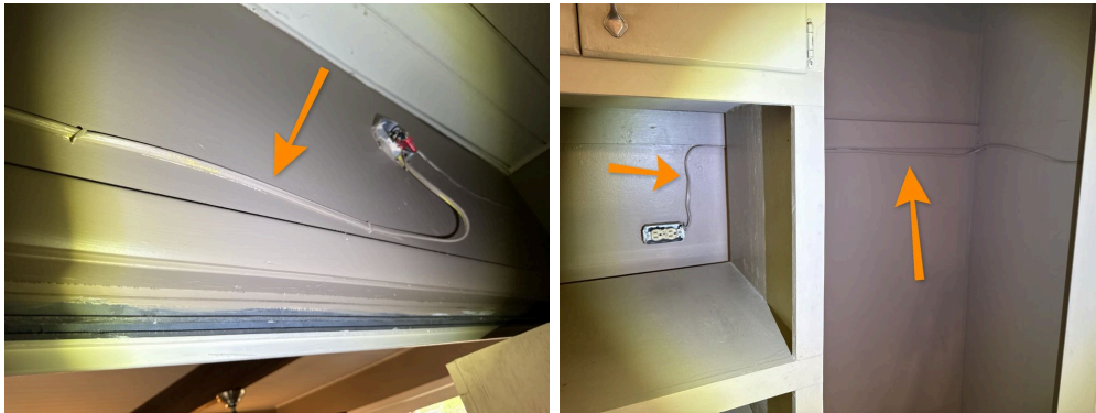
Dispose and circuit wiring noted in closet in dining area
