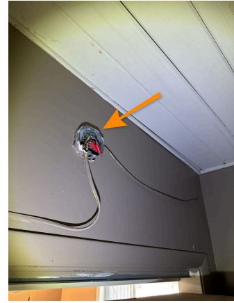
Junction box in closet in dining room
