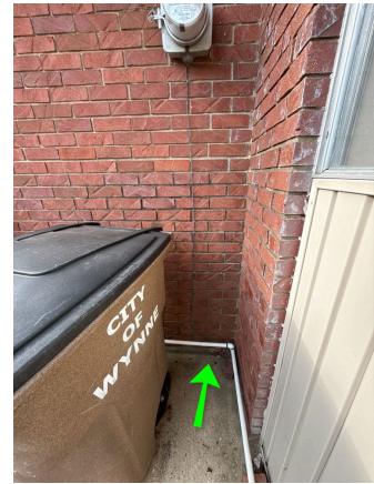
Grounding conductors disappears into the concrete and is not visible
