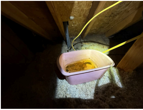
A plastic pan with noted water standing is noted near the overhead power penetration area where the roof and wall intersect.
