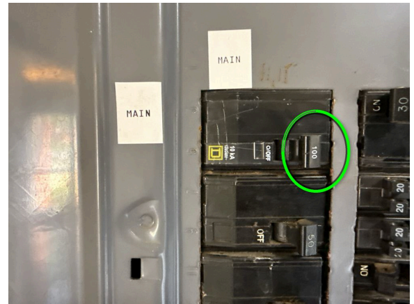
100 amp main disconnect noted
