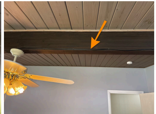
Primary bedroom ceiling fans powered by an extension cord
