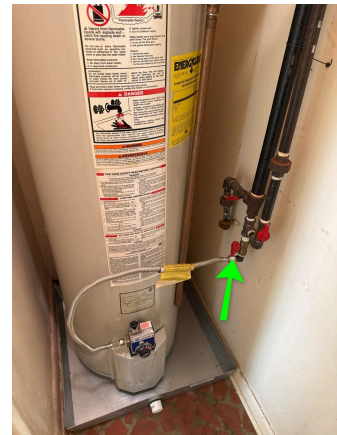
Water heater gas shut off valve
