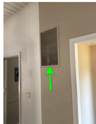
Return air vent, View
