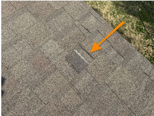
Damaged shingle with exposed fiberglass noted on east side of carport.
