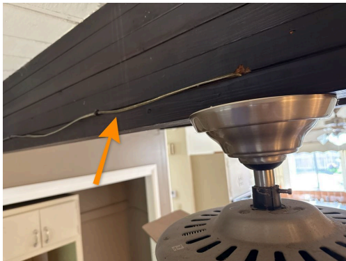
Lamp cord wiring in use for permanent installation
