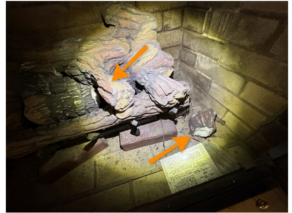
Broken decorative log piece noted
