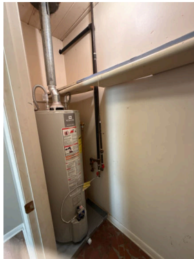
No air supply from attic noted
