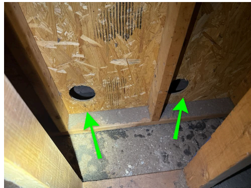
Several areas have holes drilled in some sheathing, presumably to provide some type of airflow.
