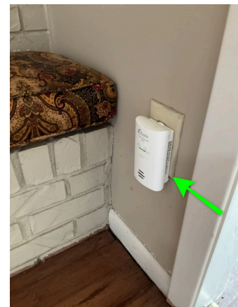
Tester located near fireplace
