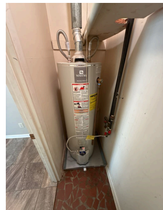
Water heater View
