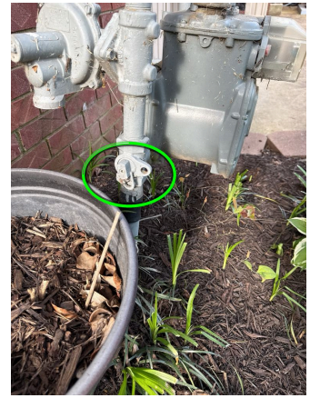
Gas shut off valve, View
