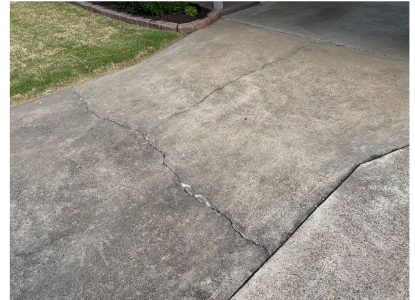
Cracking in the driveway is noted. Suggest sealing.
