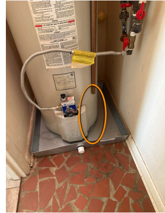
TPRV emergency drain should terminate within 6 inches of the floor.
