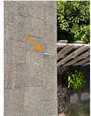
Damaged shingle with exposed fiberglass noted on east side of carport.
