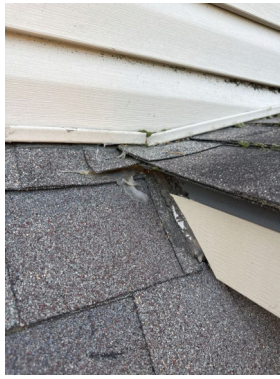
Approximate location of potential water infiltration.
