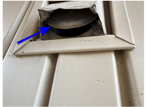
Dryer vent trap door will not close. Simple cleaning may take care of this.
