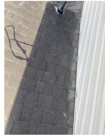
Moss growth is noted north side is shaded.
