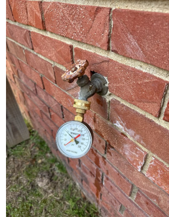
West facing faucet
