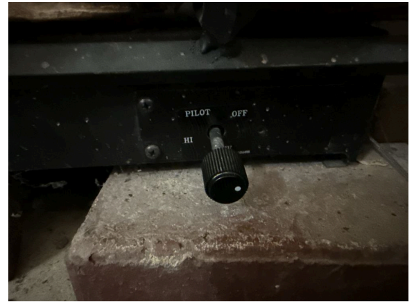
Control valve is in the off position.
