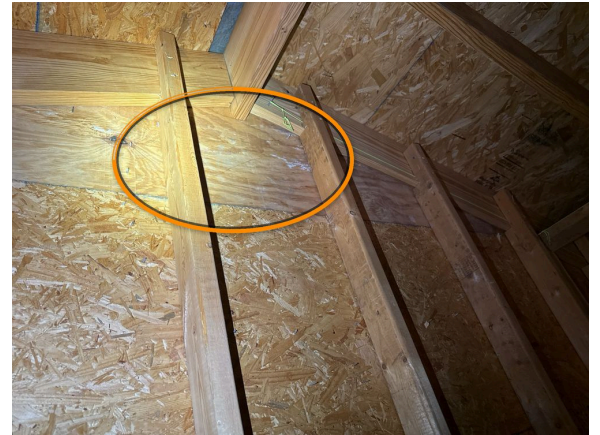
Gable vents installed on front of house are blocked. No ventilation here.
