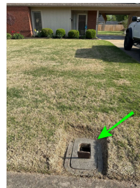
Water meter is located in front of the house near the sidewalk
