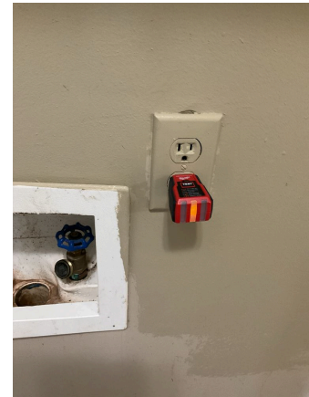
Laundry room no GFCI
