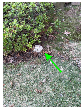
A sewer cleanout is located on the west side.
