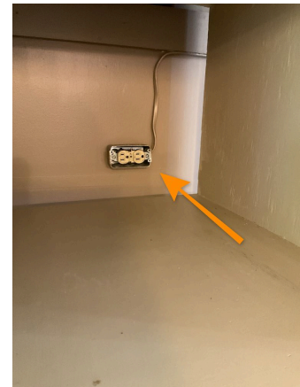
Outlet for refrigerator
