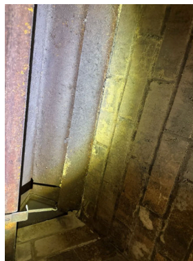
Damper appears to be abandoned. The house may have originally had a true chimney wood-burning fireplace. The chimney has been abandoned and removed
