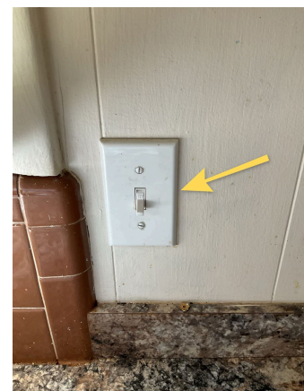
Kitchen unidentified switch noted
