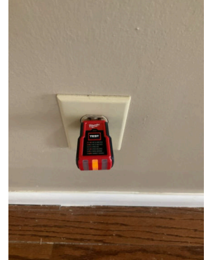
Living room ungrounded outlets noted
