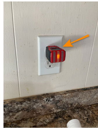
No GFI in kitchen
