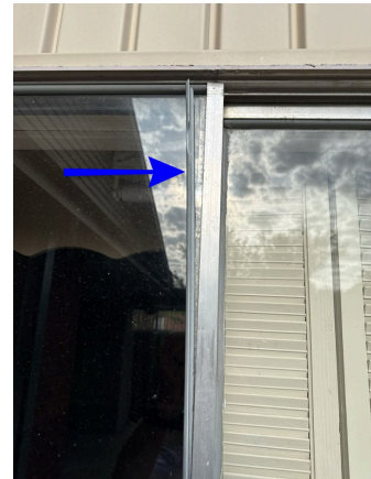
Loose glazing trim noted at kitchen window
