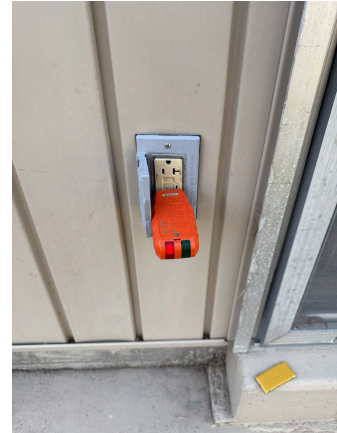
Exterior GFCI at sunroom door would not trip using the test button.
