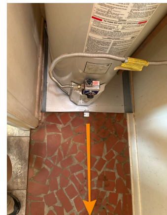
Emergency drain pan does not have a drain line to the exterior.
