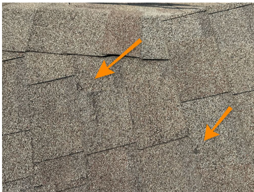
Minor damage with no penetration noted on east slope of carport
