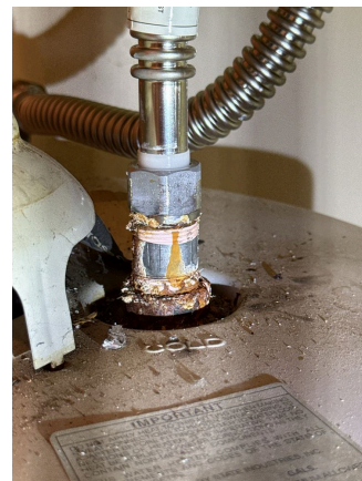
Corrosion noted at the pipe nipple to flex line connection point.
