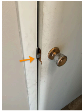
Foyer closet door not latching
