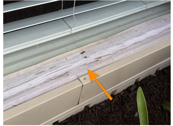
Wood trim component at front window needs to be repainted.
