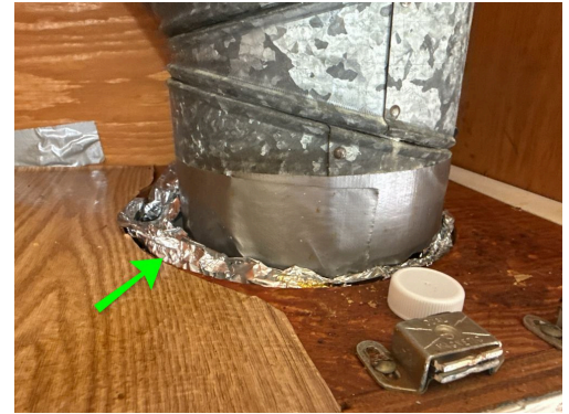
Unconventional installation noted.
