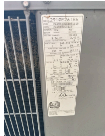
Data plate S/N# 2910E26186 manufacture date 07/2010
