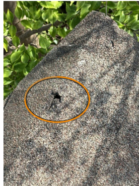
Damage shingle with penetration at the north east corner of carport.
