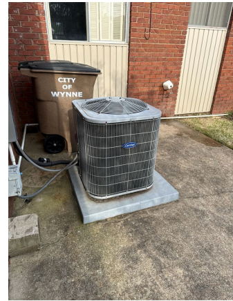
AC condenser unit
