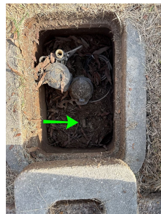
Main wall shut off is located at the water meter
