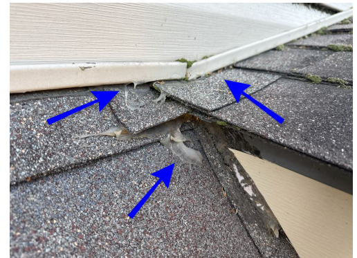
Sealant has been installed in multiple locations at this intersection. Note see flashing comment for water penetration.
